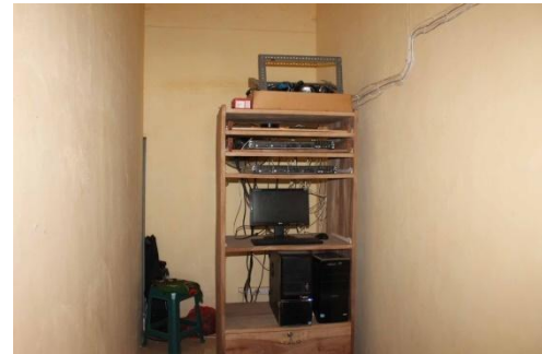
Gambar 2. Survey Kesiapan Ruang Server Internet
