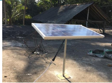
Gambar 3. Instalasi panel surya di atap Masjid PP. Nurussalam
