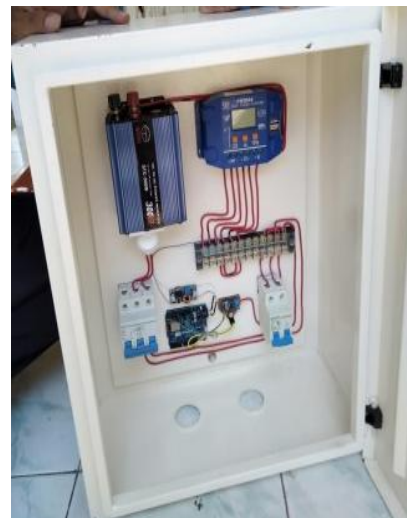
Gambar 4. Rangkaian Solar charge controller , inverter, MCB AC 2 Amphere, terminal ke beban dan sambungan sistem IoT
